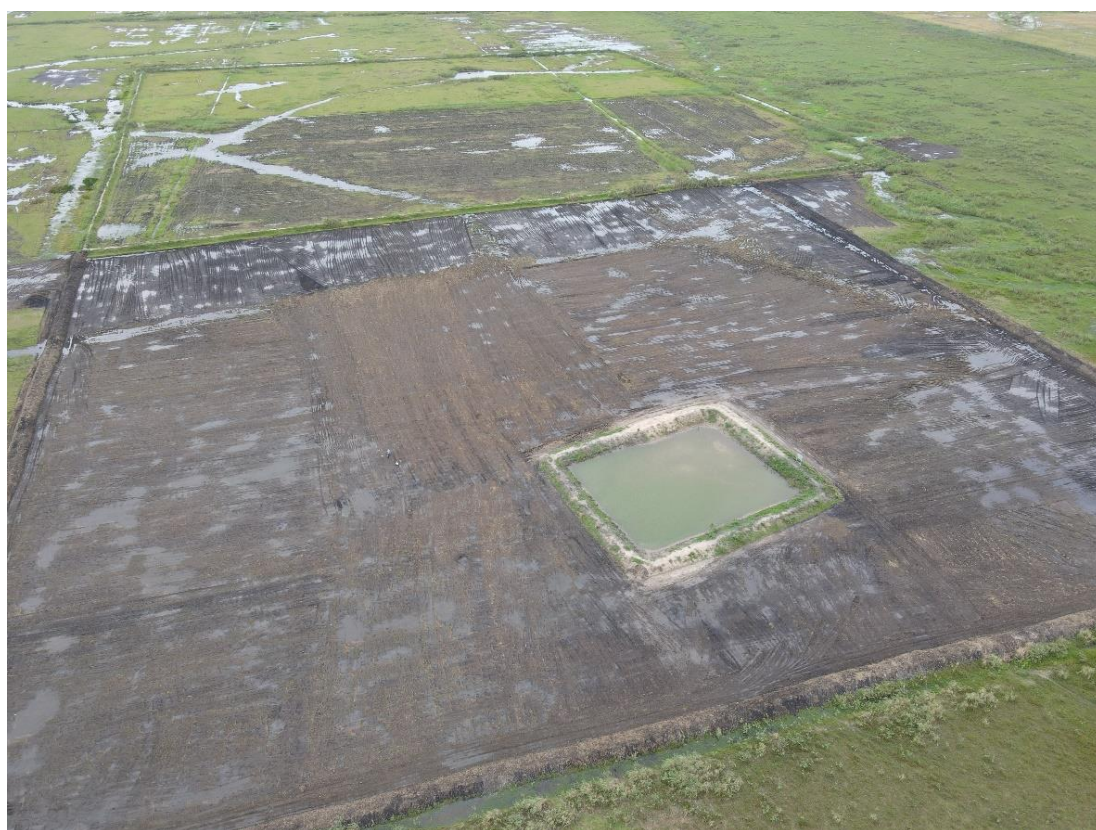
Photograph 9. Aerial photograph showing the area enhanced by ground lowering (foreground), surrounded by the new bund, and area ploughed inside the existing water control plot (background)
